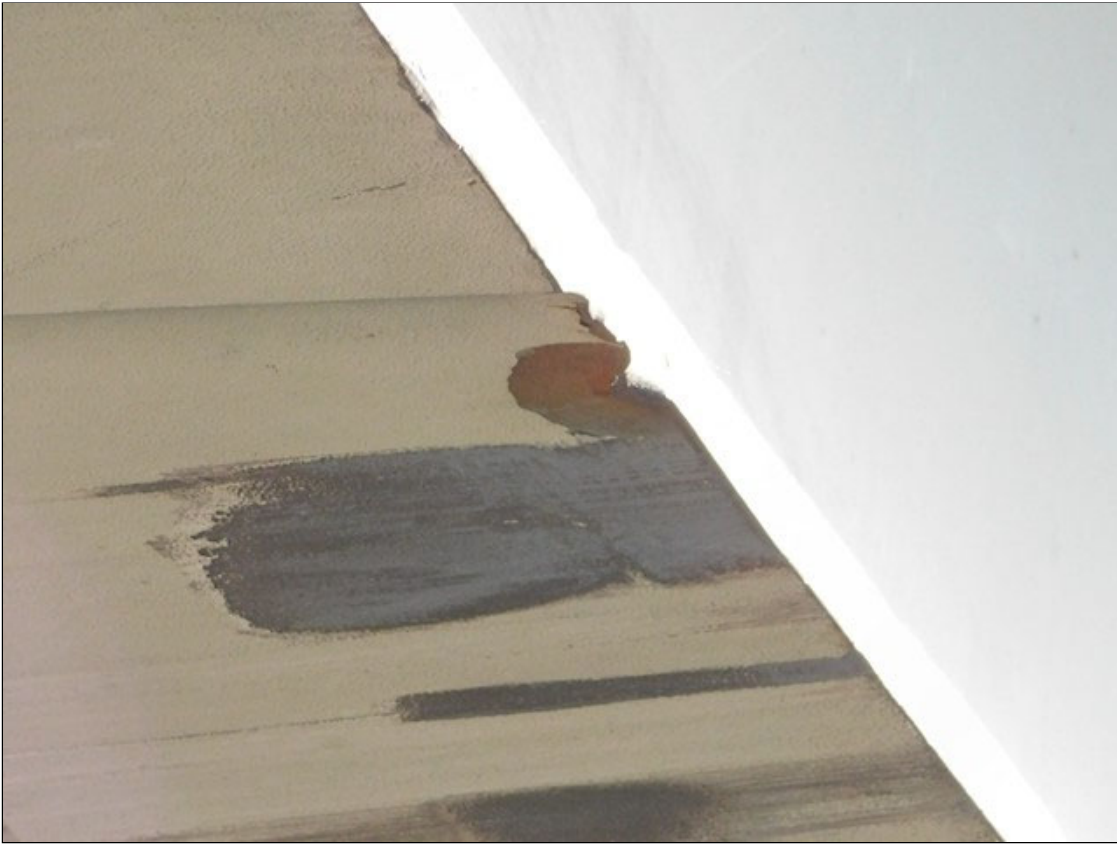
SPAN 2 Beam 5: (PAR) DAMAGE TO BOTTOM FLANGE APPROXIMATELY 25 FEET FROM BENT 2, UP TO 2 INCH DIAMETER GOUGE ON SOUTH EDGE AND UP TO 1/2 INCH DISTORTION TO BOTTOM WEB
