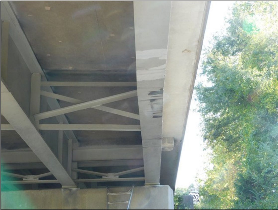
SPAN 2 Beam 5: 12 FEET X 1/2 INCH DISTORTION FROM IMPACT DAMAGE ON BOTTOM FLANGE AND WEB STARTING 25 FEET FROM BENT 2 (PAR)
