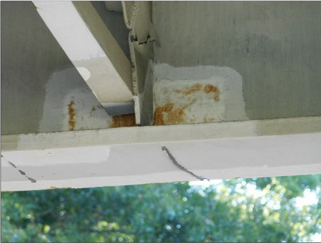
SPAN 2 Beam 5: (2025 NO HANDS-ON ACCESS) 5-1/4 INCHES LONG HORIZONTAL CRACK IN WEB ABOVE BOTTOM FLANGE AT 37 FEET FROM BENT 2 BEARING (PAINT APPLIED) (PAR)
